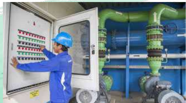
Fasilitas Pengolahan Air Bersih Clean Water Treatment Plant
