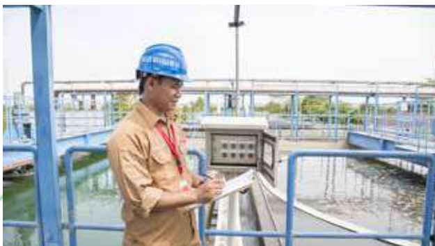
Fasilitas Pengolahan Air Limbah Waste Water Treatment Plant
