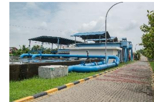
Clean Water Treatment Plant (Looping System Pipe)
